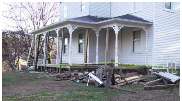
At the Reeves farm house, interim repairs are underway to shore up the deteriorated front porch.
